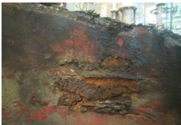
Fig. 2 Heavily corroded scrubber pipe.
