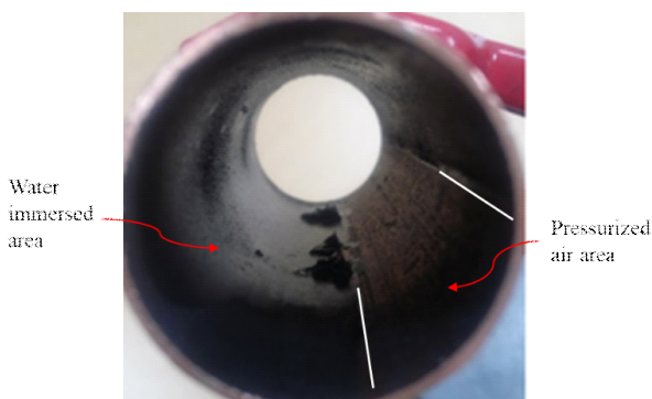
Fig. 1 Inner surface of a failed copper sprinkler tube with mounds of corrosion by-products formed near the water-air line.
