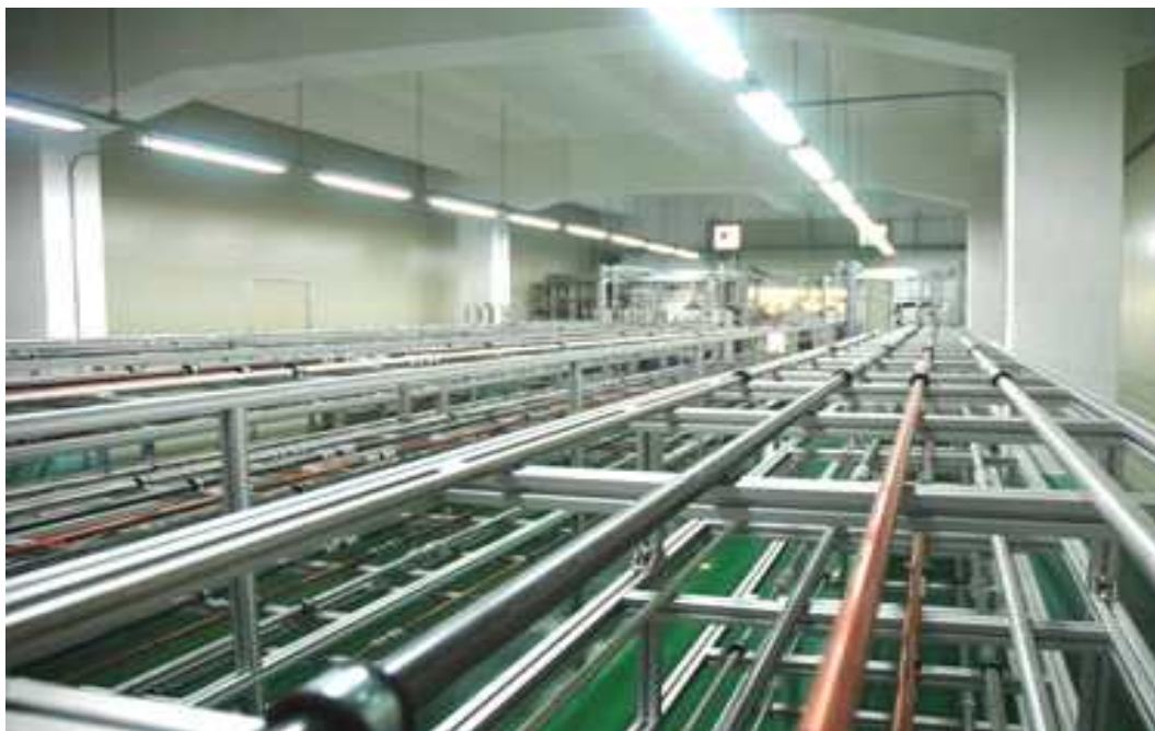
Fig. 3. Test pipes in demo plant consisting of carbon steel, copper, galvanized iron, cast iron.
