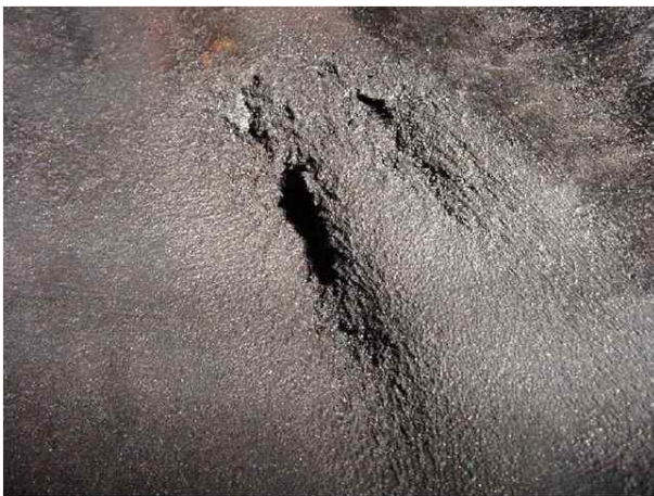
Fig. 2. Damaged Surface by LDIE 2,3) .
