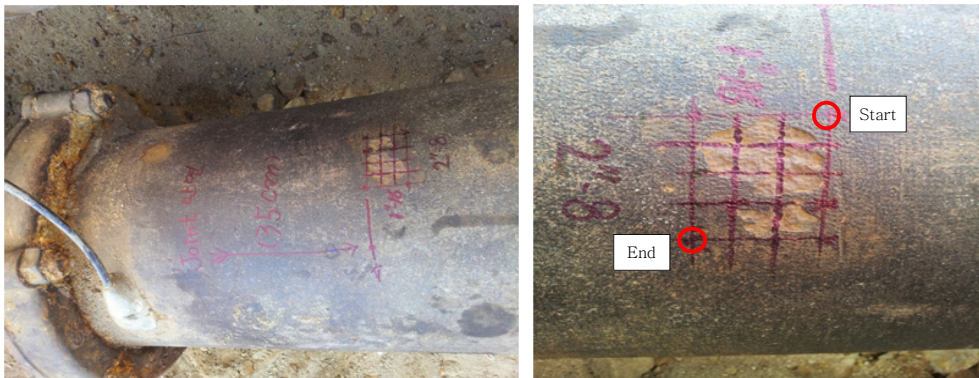
Fig. 5. Picture of damaged pipe.
