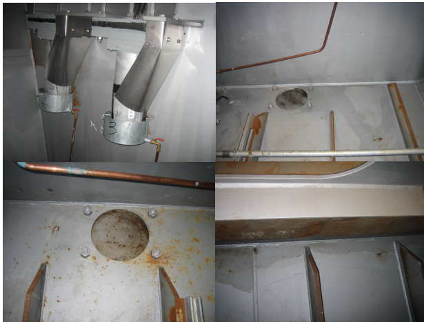
Fig. 15. Corrosion Occurred in Hanger Rope Anchorage Section.
